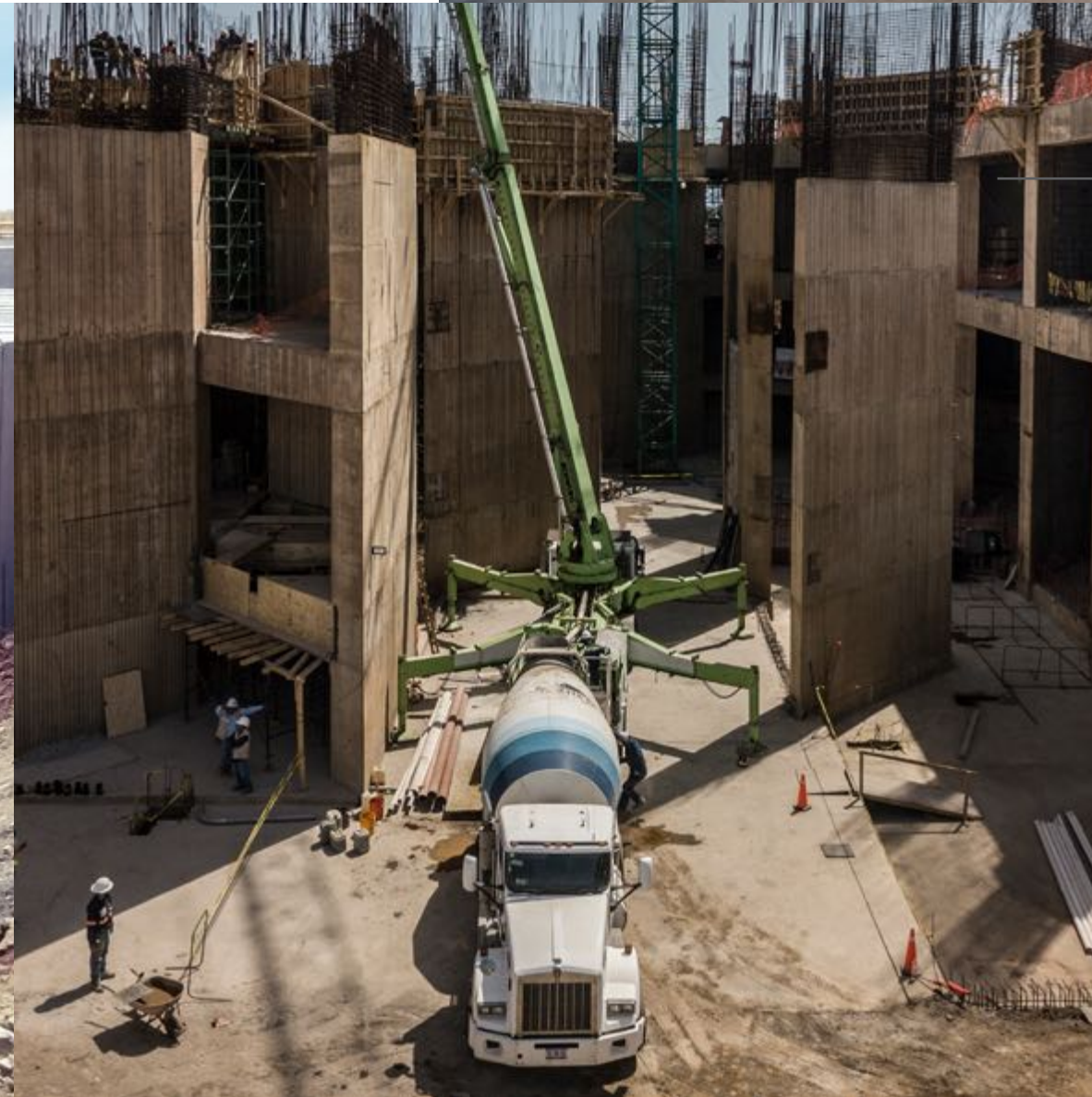
PREMIXED CONCRETE SUPPLY F'C 350 KG/CM 2 ON 28 DAYS, ADDITION OF 10 MM, REV. 16 CM WITH BROWN MOKA PIGMENTATION AND PUMPED TO 42 M WITH TELESCOPIC BOOM PUMP.
