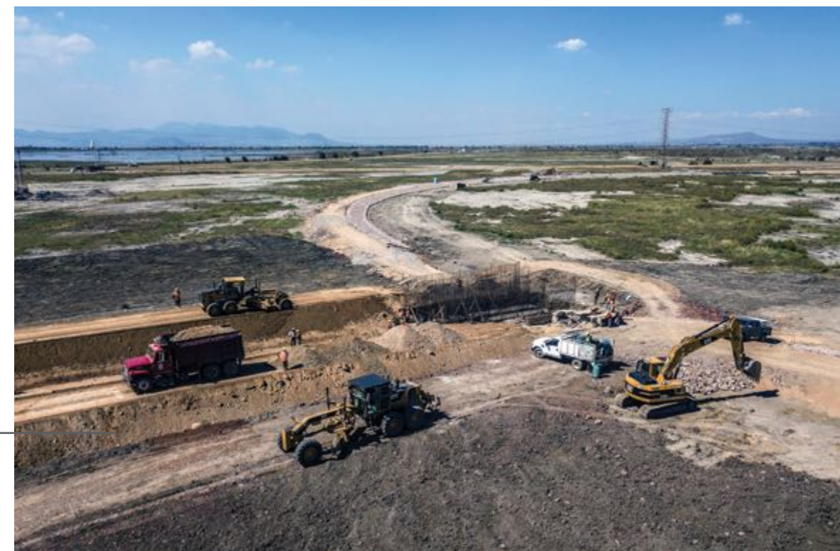
CONSTRUCTION OF DISCHARGE CANAL TO DREN CHIMALHUALCAN II, COATED WITH REINFORCED CONCRETE, TEXCOCO, STATE OF MEXICO.
