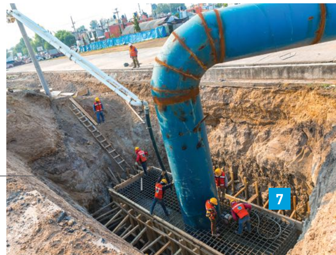
INSTALLATION OF A 60" DIAMETER WELDING STEEL PIPELINE, METROPOLITAN LINE, TULTEPEC, STATE OF MEXICO
