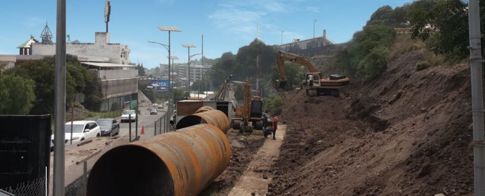
STEEL PIPES FOR SLEEVES 3.02M IN DIAMETER, INTERLOMAS, HUIXQUILUCAN, STATE OF MEXICO
